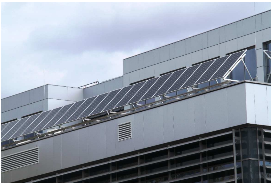
Fig. 4.21. PV panels located on the roof of an office building
